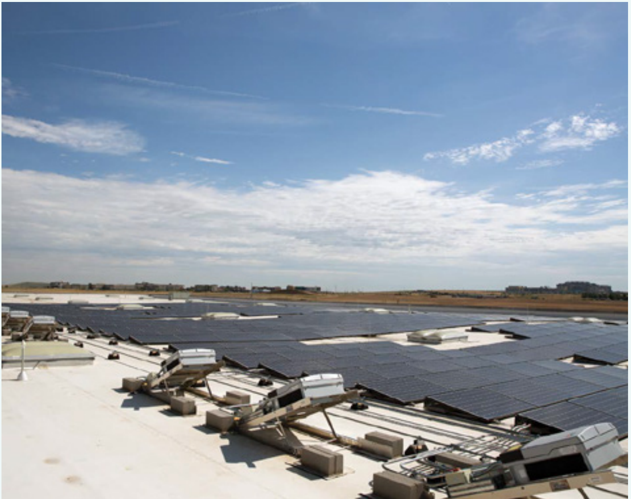
Looking out from the Panasonic rooftop, a canopy of solar panels covers a city-owned parking lot as part of the facility's onsite microgrid.
